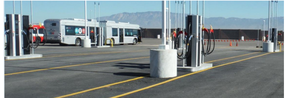
Figure 3-1. A Plug-in Charging Yard | Source: WSP
